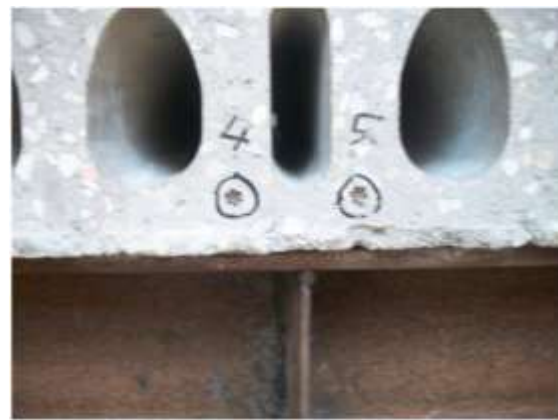
Figure 11: Anchorage failure of the two middle strands in SA
